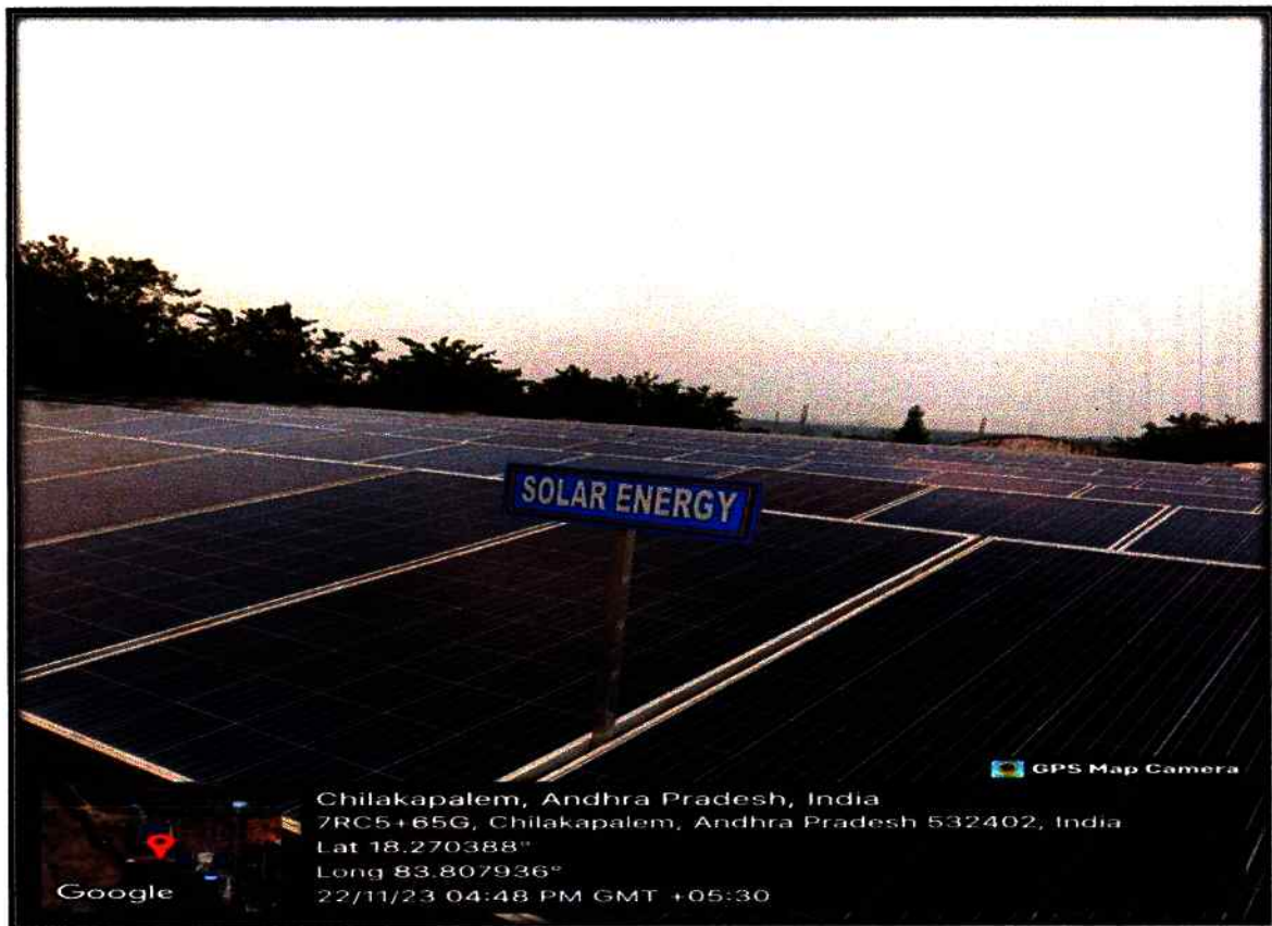
Roof Top Solar Energy Generation
